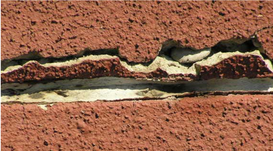
Figure: Block of flats type T 06 B. on Lučenecká street – degradation of gable panel insulation
