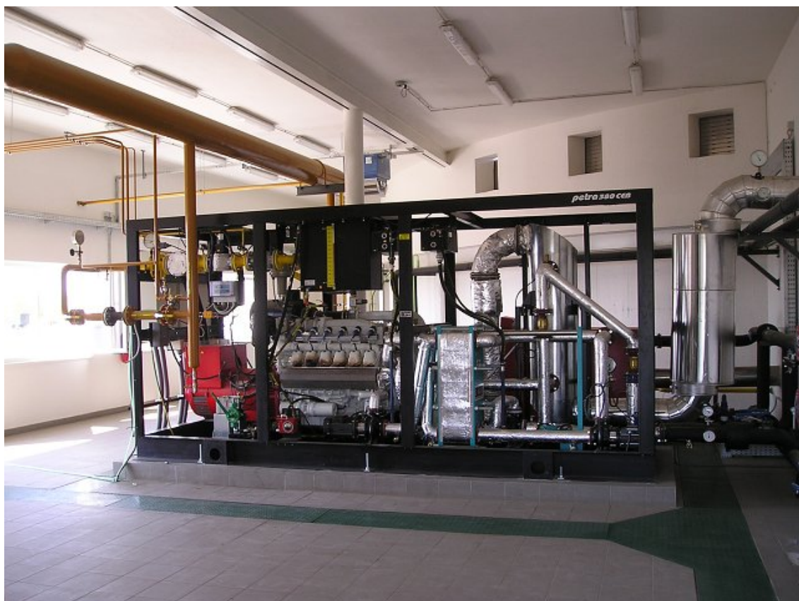
Figure: CHP unit in biogas plant Hurbanovo
